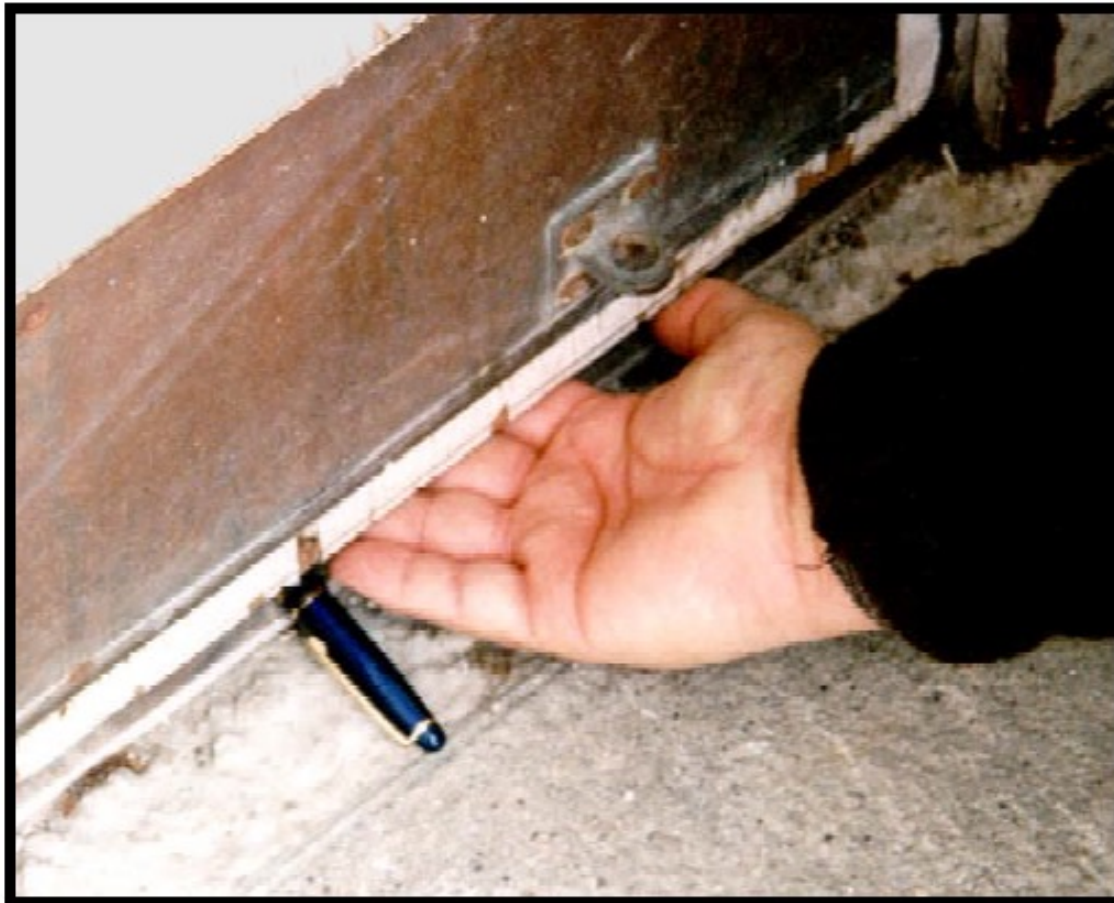
Figure 10: This gap at the bottom of the door is large enough to allow rat and mouse access to the building. Installation of a door sweep would exclude rodents.
